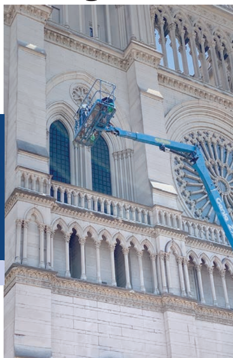
A contractor is lifted up the Cathedral Basilica of the Assumption's façade on the side of Madison Avenue, Covington, to assess a gargoyle for damage.
